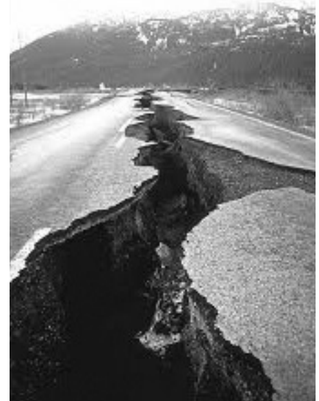
A crack developed in this highway, believed to be near Portage. (USGS photo)
